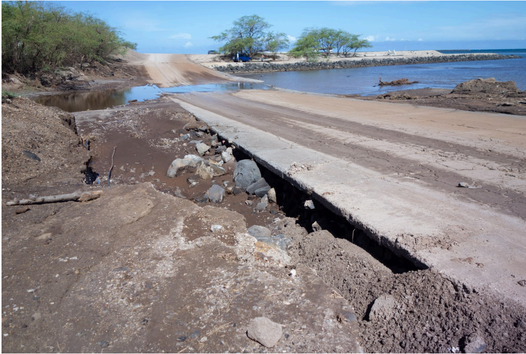
Paved access to Coral Flats is inundated with sediment and erosion from the 5/10/2024 flashfloods.
