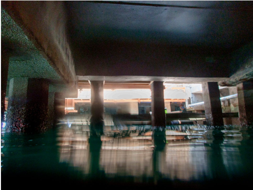
Opening at structural floor/deck construction at Pier 2, Kawaihae Harbor , 4/3/2025
