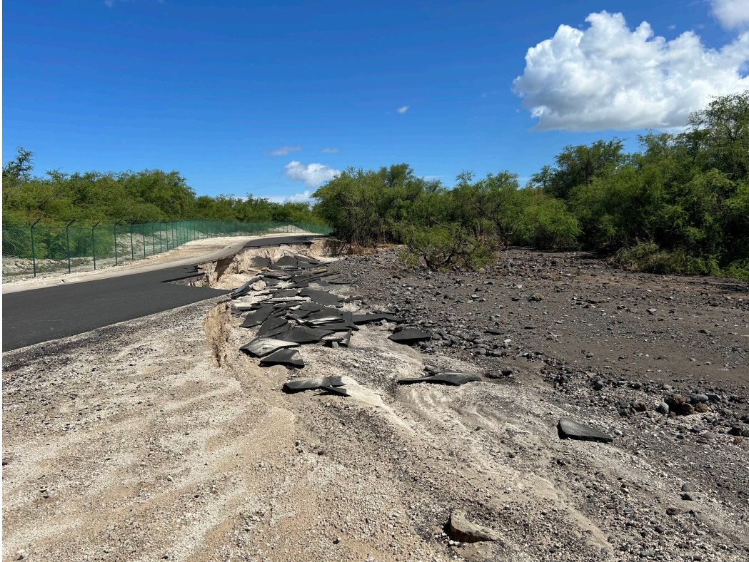
Road to Small Boat Harbor South damaged from 5/10/2024 flashfloods
